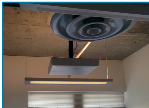
Figure 10: xArray Installed Slightly Lower Than Vents and Lighting
